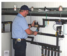
Greg White, MEPS field manager, completes the installation of a commercial boiler system.
