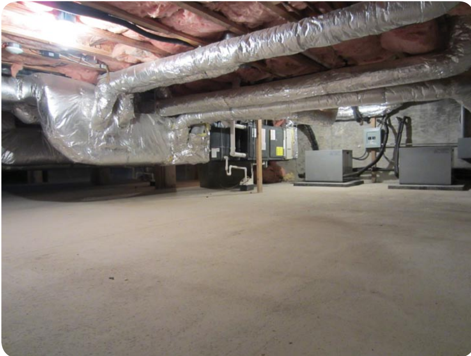
A view of the basement area occupied by the heat pumps and associated ductwork.
