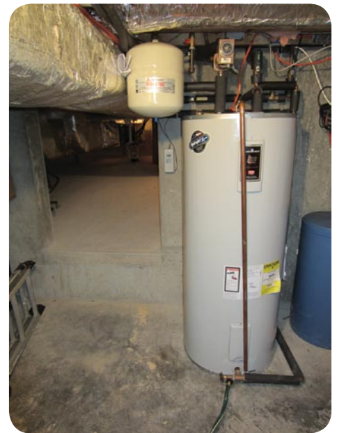
The solar-powered water heater in the Randels' basement.
