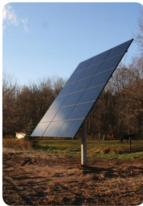
The solar panel is installed right at the edge of the same farm field as the turbine.
