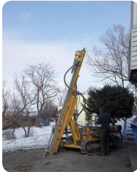
This machine drilled eight vertical holes 70 feet deep for the geothermal tubing.
