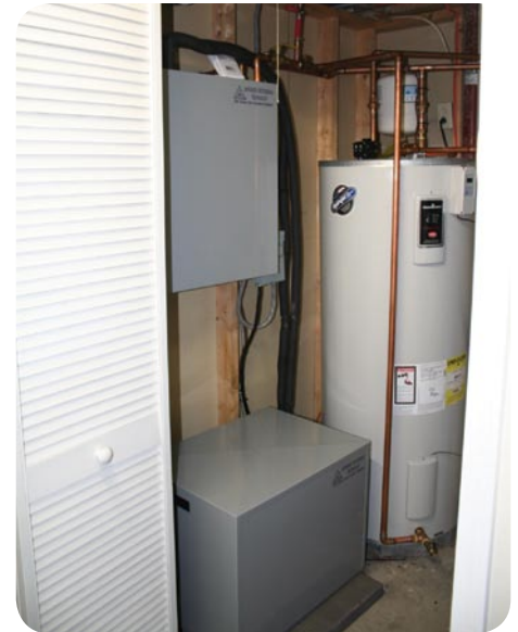
Geothermal heat pump and domestic water heater are in the basement.
