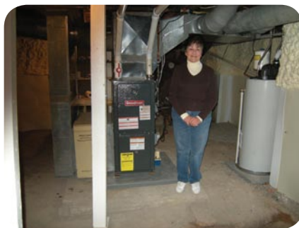
Anna with her new furnace, water heater and high efficiency air filter.
