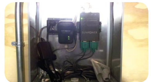
System monitoring area.
