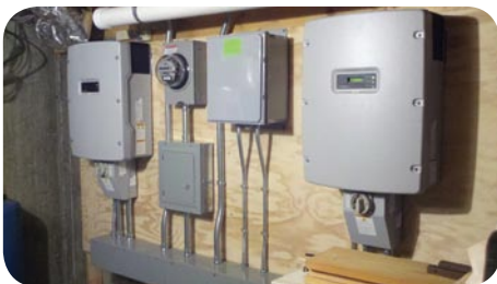
The inverters are mounted on the basement wall.
