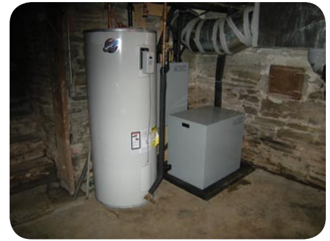
The geothermal heat pump, solar electric water heater and some of the new ductwork.
