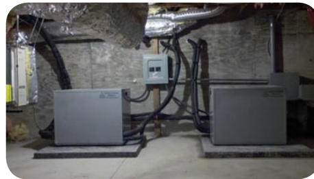
Close-up of heat pump area.
