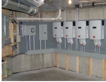
Solar system control panel.
