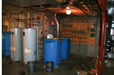
Geothermal water heaters and hydronic boilers systems.
