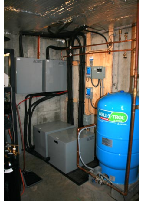
The geothermal overflow tank and heat pumps.
