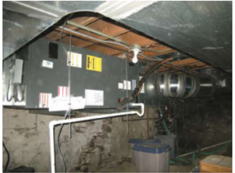
Maneuvering this large air handler and ductwork into the basement and installing it was the job's major hurdle.
