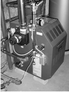
The Davias' new Williamson boiler.
