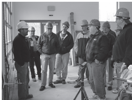
The tour checked out the truck bay system. HVAC students from BOCES #1 got an up close lesson in commercial installation when they toured the new Bushnell's Basin firehouse on Kreag Road, just north of Route 96.
