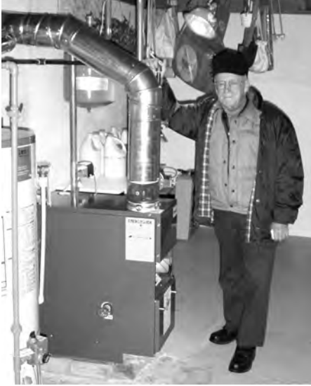
Joe Masetta shows off his new boiler.
