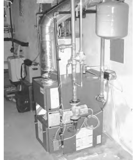
The control side of Joe's new boiler.
