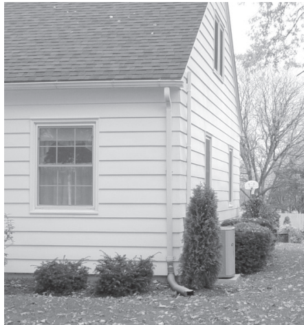
The Carrier A/C compressor on the side of the house is nearly hidden by a tree.
