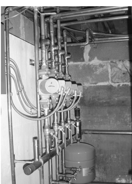
The manifold system - four zones plus a spare for future expansion.
