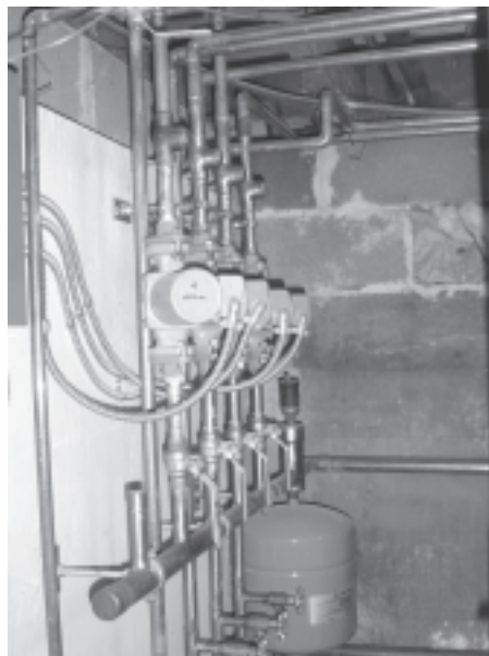
The manifold system - four zones plus a spare for future expansion.
