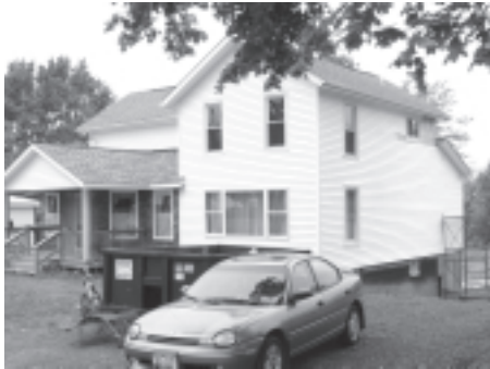
The finishing touches are still being done to the Ritchie's remodeling project...
