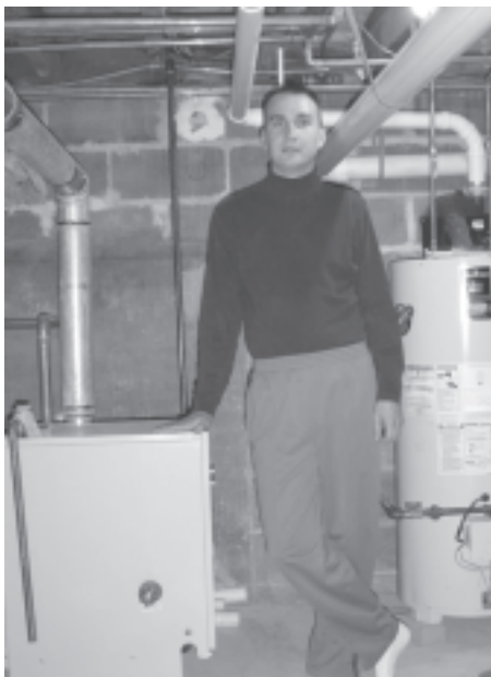
Scott Ritchie stands between his new boiler and water heater.
