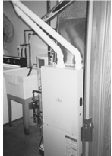
Tom is pleased with his new high efficiency furnace and hot water heater.
