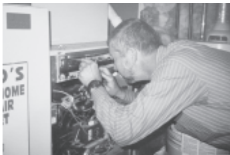
HVAC technician Steve Andrews checks the burners of a furnace during the cleaning and tune-up process.
