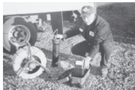
Plumber Jim Perry feeds the SeeSnake into a pipe while he checks condition of the pipe by viewing the small television monitor.
